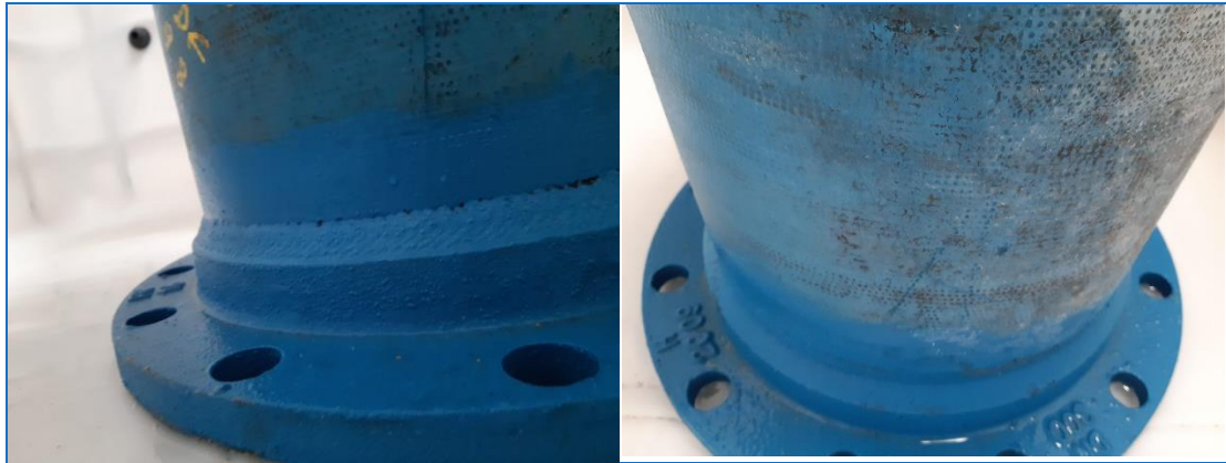
Figure 7 & 8 flanged ends with 100mm of QD8 coating up the barrel from bottom of pipe standing on the tank floors after tanks drained
