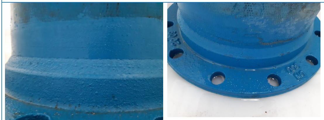
Figure 9 & 10 close up of flanged ends with 100mm of QD8 coating up the barrel from bottom of pipe standing on the tank floors after tanks drained – some rust spots / loose coating visible
