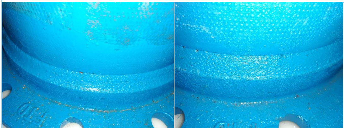
Figure 11 & 12 close up with flash of flanged ends with 100mm of QD8 coating up the barrel from bottom of pipe standing on the tank floors after tanks drained – some rust spots / loose coating visible
